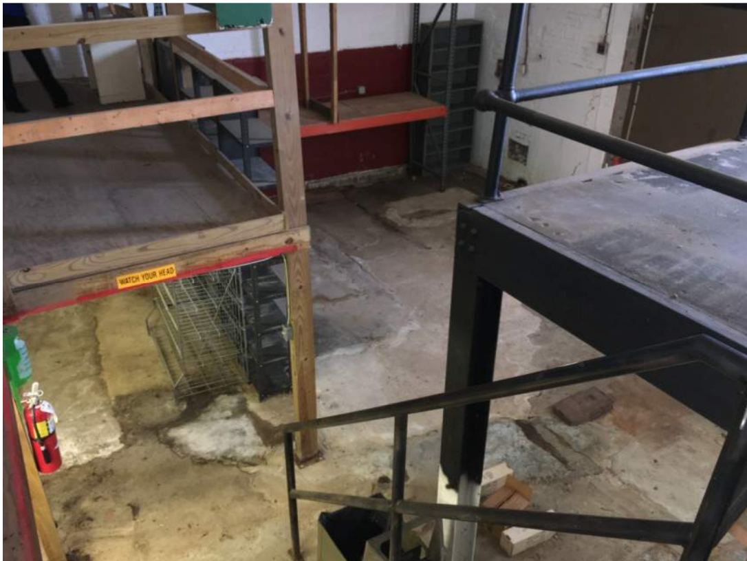
Photo 34: Lower Level North Room, Viewed from Staircase at Southwest Corner of Room
