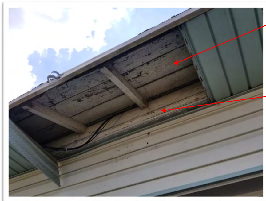
Photograph #0001 Silver Lead-Based Paint associated with metal roofs of East and West Buildings
