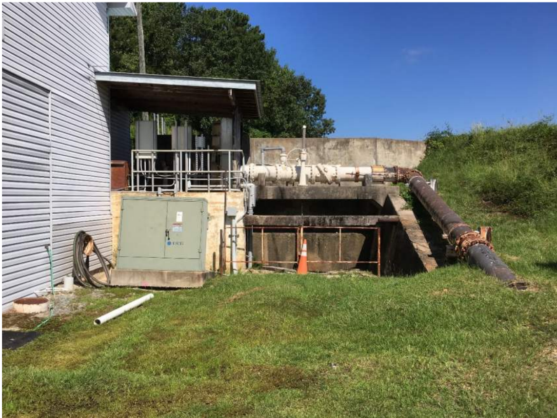
Photo 10: Wet Well, Intake Retaining Wall, Electrical Cabinet and 16-inch Raw Water Line, Viewed from South
