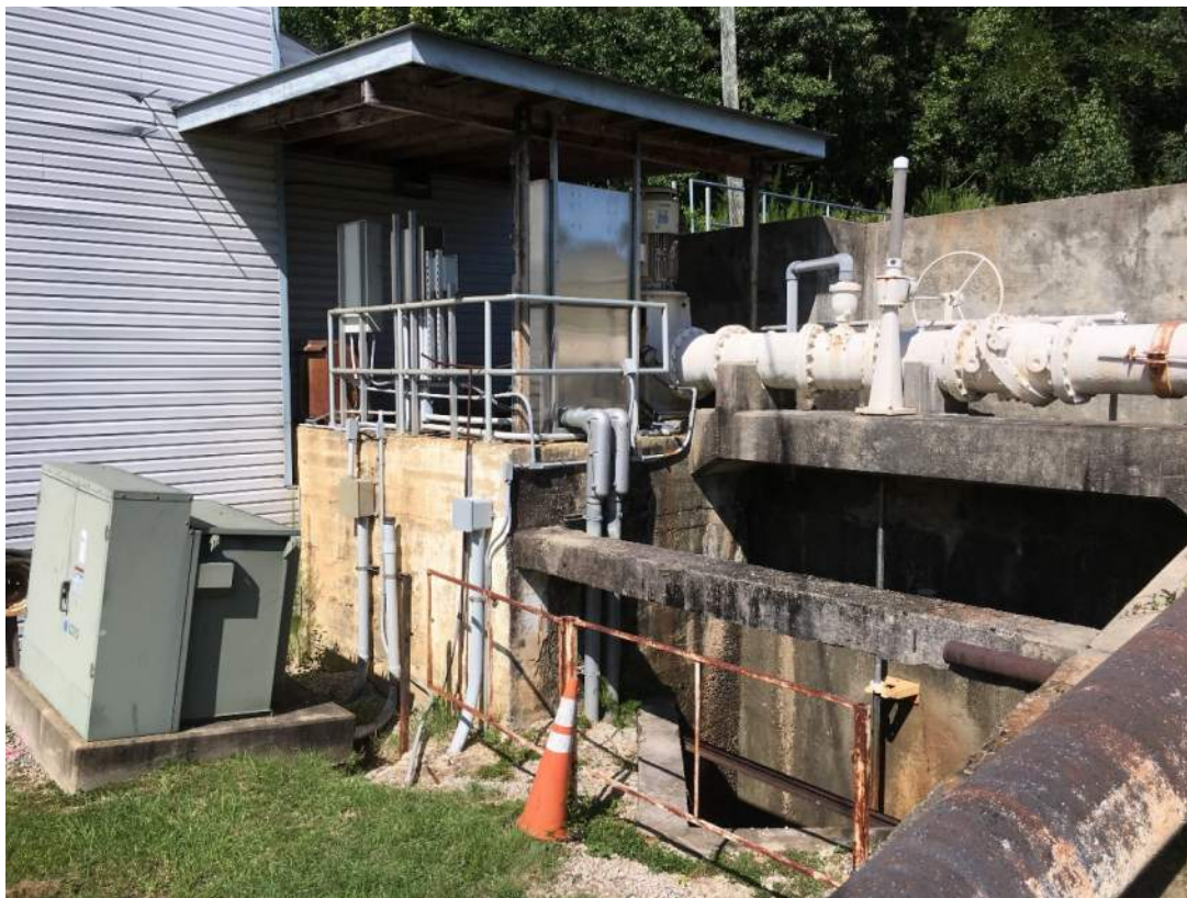
Photo 11: Wet Well, Intake Retaining Wall, Electrical Cabinet and 16-inch Raw Water Line, Viewed from East
