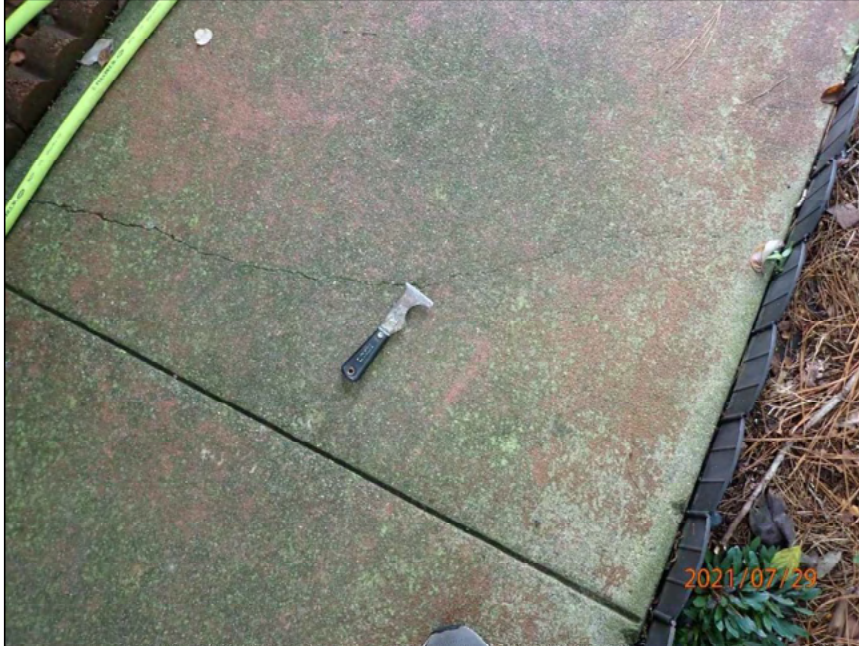
Photo 5 Cracks in concrete walkway
