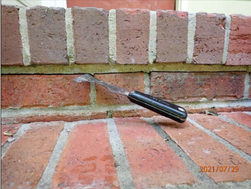
Photo 7 Horizontal crack for full length of front porch
