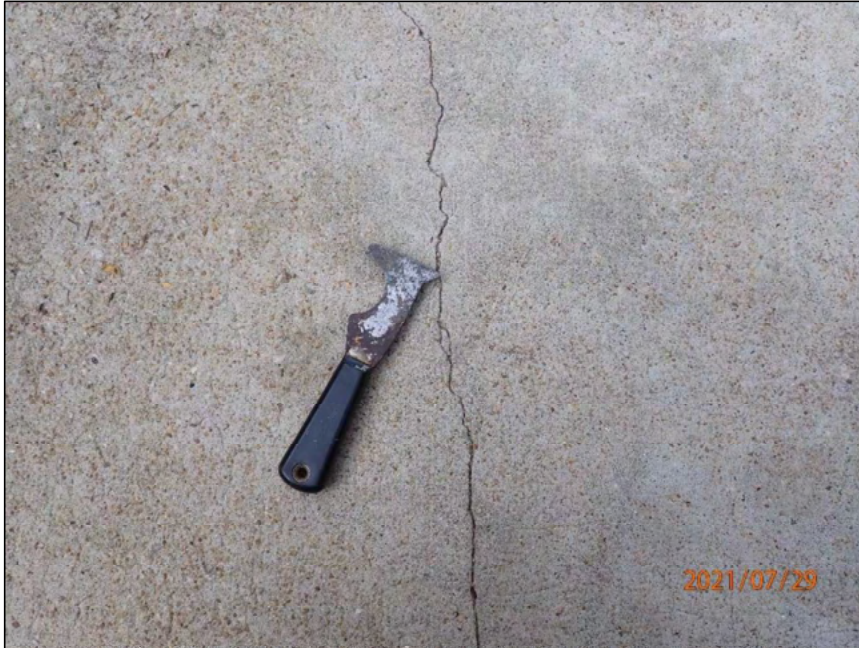
Photo 5 Cracks in concrete driveway
