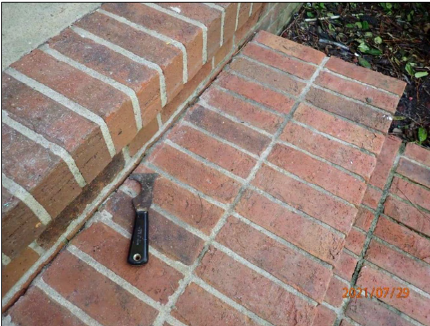
Photo 8 Separation crack at stairs
