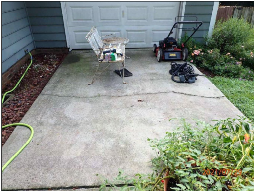
Photo 6 Cracks in concrete driveway
