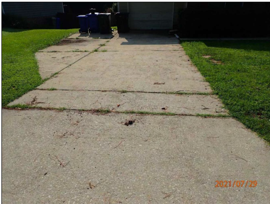
Photo 6 Cracks in concrete driveway
