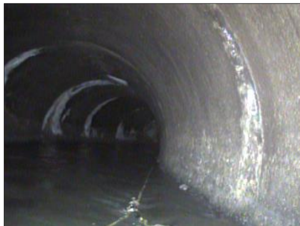
Photo: PWC-2103892-01-AMH '016462'-AMH '016461'-LR at 690.8 ft.JPG, 00:40:26 690.8FT, Alignment Right, 25°
