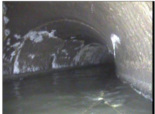
Photo: PWC-2103892-01-AMH '016462'-AMH '016461'-LR at 521.0 ft.JPG, 00:27:37 521FT, Alignment Right, 25°
