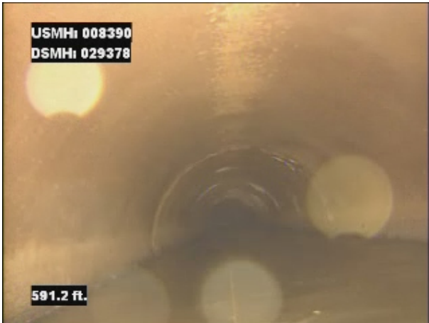
Photo: 008390_D_029378_SRV_591.jpg, VCR No.: 1 591FT, Surface Reinforcement Visible, from 08 to 04 o'clock, within 8 inches of joint: NO, Finish
