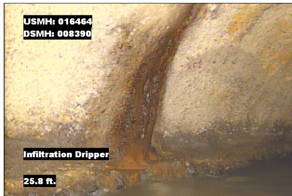
Photo: 016464_D_008390_ID_25.8.jpg, VCR No.: 1 25.8FT, Infiltration Dripper, from 09 to 11 o'clock, within 8 inches: YES
