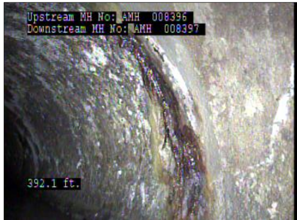
Photo: PWC-2103892-01-AMH '008396'-AMH '008397'-IS at 392.0 ft.JPG, 00:20:09 392FT, Infiltration Stain, from 01 to 04 o'clock, within 8 inches: NO
