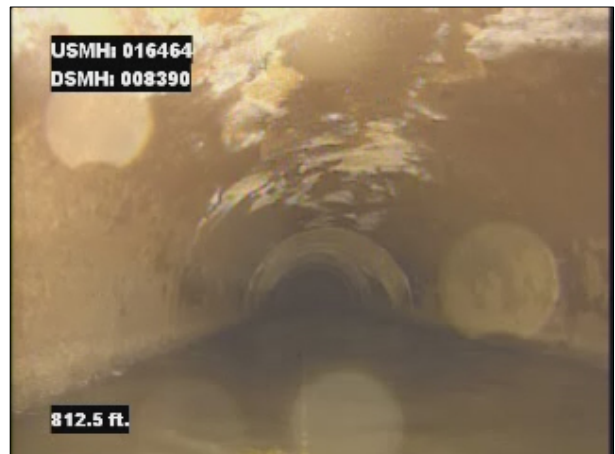
Photo: 016464_D_008390_SRV_812.jpg, VCR No.: 1 812FT, Surface Reinforcement Visible, from 08 to 04 o'clock, within 8 inches of joint: NO, Finish
