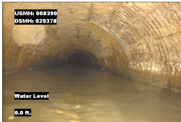
Photo: 008390_D_029378_MWL_0.jpg, VCR No.: 1 0FT, Water Level, 45% of cross sectional area
