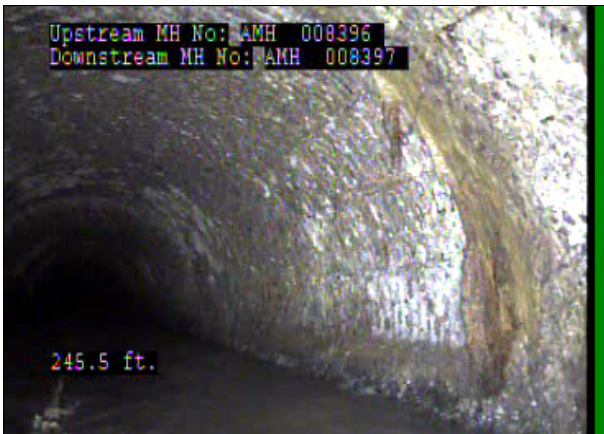
Photo: 008396_D_008397_IS_245.4_11_A.jpg, 00:10:37 245.4FT, Infiltration Stain, from 02 to 04 o'clock, within 8 inches: NO
