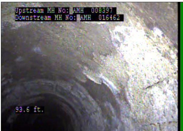
Photo: 008397_D_016462_SRC_93.5_25_A.jpg, 00:05:10 93.5FT, Surface Reinforcement Corroded, from 08 to 04 o'clock, within 8 inches: NO
