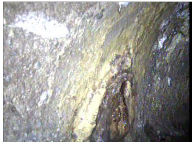
Photo: PWC-2103892-01-AMH '008396'-AMH '008397'-IS at 429.8 ft.JPG, 00:22:25 429.8FT, Infiltration Stain, at 08 o'clock, within 8 inches: NO
