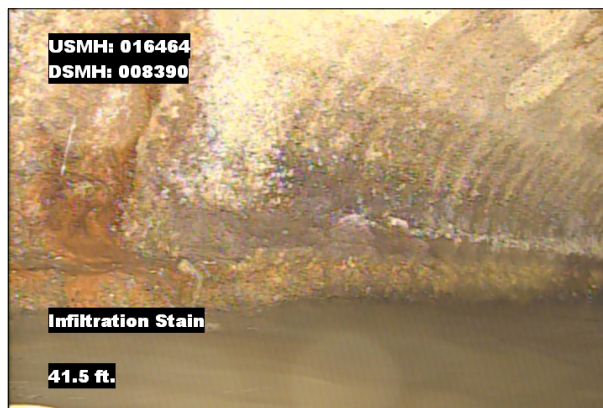
Photo: 016464_D_008390_IS_41.5.jpg, VCR No.: 1 41.5FT, Infiltration Stain, from 09 to 11 o'clock, within 8 inches: YES
