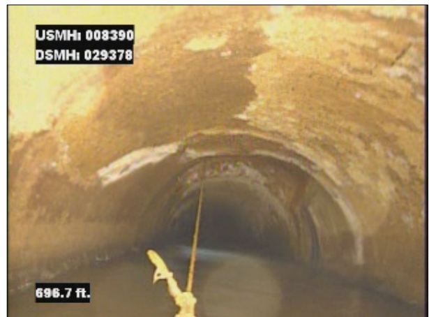
Photo: 008390_D_029378_SRV_698.jpg, VCR No.: 1 698FT, Surface Reinforcement Visible, from 08 to 04 o'clock, within 8 inches of joint: NO, Finish
