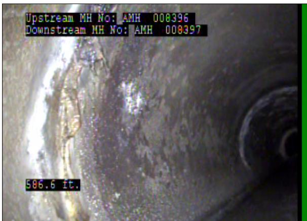
Photo: 008396_D_008397_DAE_586.6_17_A.jpg, 00:31:58 586.6FT, Deposits Attached Encrustation, 5% of cross sectional area, from 08 to 11 o'clock, within 8 inches: NO
