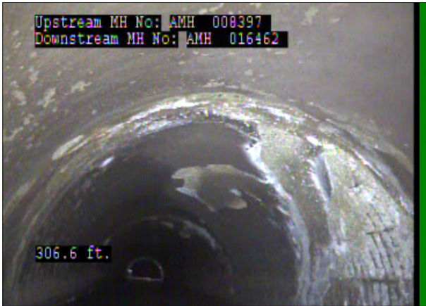
Photo: 008397_D_016462_SRC_306.6_160_A.jpg 306.6FT, Surface Reinforcement Corroded, from 01 to 05 o'clock, within 8 inches of joint: YES
