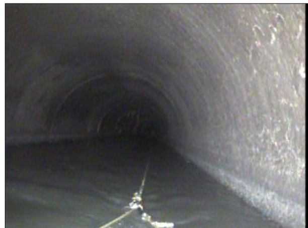
Photo: PWC-2103892-01-AMH '016462'-AMH '016461'-SRI at 651.5 ft.JPG, 00:37:19 651.5FT, Surface Roughness Increased, from 08 to 04 o'clock, within 8 inches: NO
