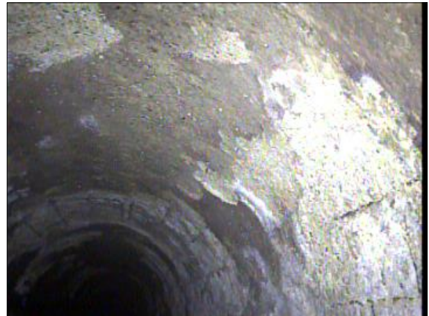
Photo: PWC-2103892-01-AMH '008397'-AMH '016462'-SAV at 93.4 ft.JPG, 00:04:11 93.4FT, Surface Aggregate Visible, from 08 to 04 o'clock, within 8 inches: NO
