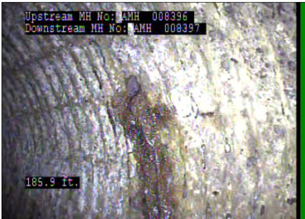
Photo: 008396_D_008397_IS_185.9_10_A.jpg, 00:08:21 185.9FT, Infiltration Stain, from 03 to 04 o'clock, within 8 inches: NO
