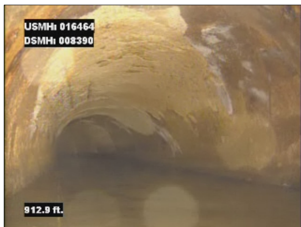
Photo: 016464_D_008390_DAE_912.jpg, VCR No.: 1 912FT, Deposits Attached Encrustation, 5 %of cross sectional area, from 08 to 04 o'clock, , within 8 inches of joint: YES
