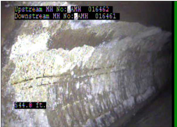
Photo: 016462_D_016461_SRC_544.8_42_A.jpg, 00:30:28 544.8FT, Surface Reinforcement Corroded, from 08 to 11 o'clock, within 8 inches: NO
