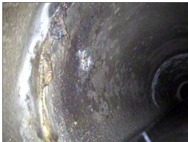
Photo: PWC-2103892-01-AMH '008396'-AMH '008397'-DAE at 586.6 ft.JPG, 00:31:58 586.6FT, Deposits Attached Encrustation, 5% of cross sectional area, from 08 to 11 o'clock, within 8 inches: NO
