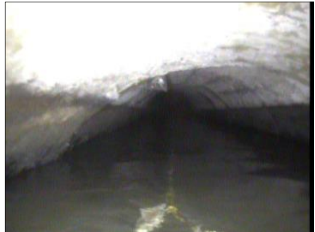
Photo: PWC-2103892-01-AMH '016461'-AMH '016460'-LL at 83.0 ft.JPG, 00:05:02 83FT, Alignment Left, 25°
