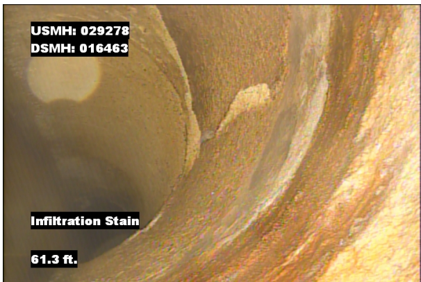
Photo: 029378_D_016463_IS_61.3.jpg, VCR No.: 1 61.3FT, Infiltration Stain, from 08 to 04 o'clock, within 8 inches: NO
