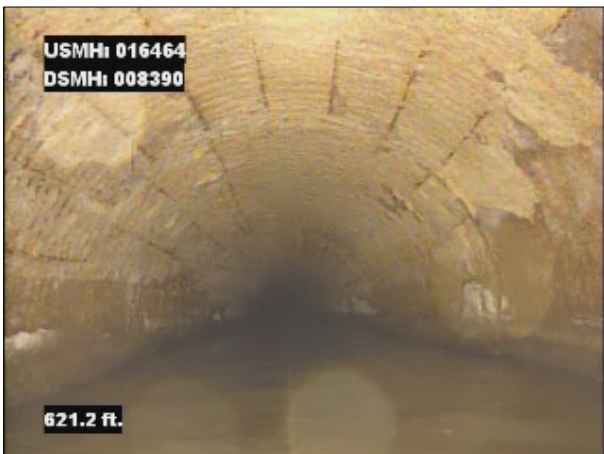
Photo: 016464_D_008390_SRV_621.jpg, VCR No.: 1 621FT, Surface Reinforcement Visible, from 08 to 04 o'clock, within 8 inches of joint: NO, Finish
