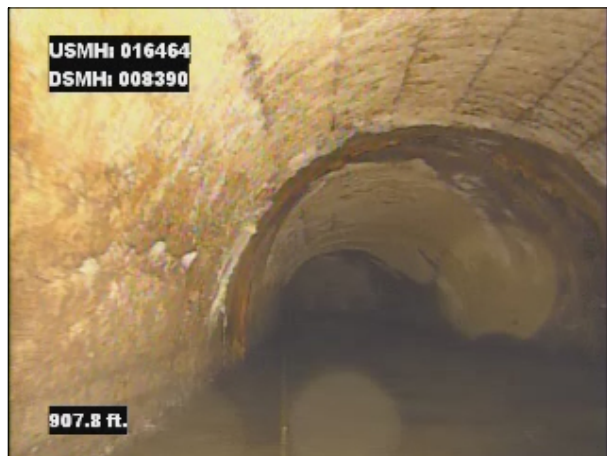
Photo: 016464_D_008390_IS_907.jpg, VCR No.: 1 907FT, Infiltration Stain, from 08 to 04 o'clock, within 8 inches of joint: YES
