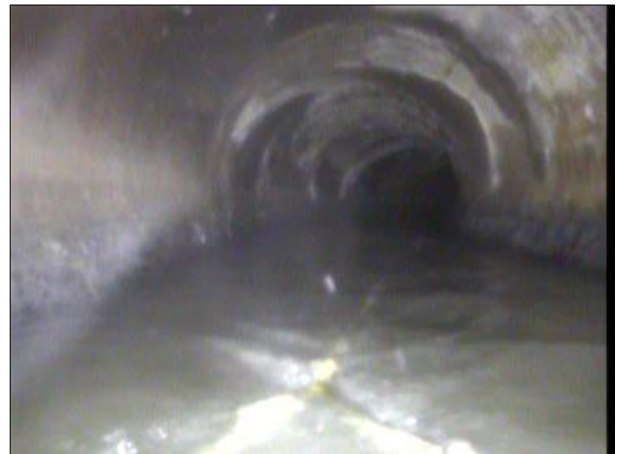
Photo: PWC-2103892-01-AMH '016461'-AMH '016460'-LR at 183.6 ft.JPG, 00:08:35 183.6FT, Alignment Right, 15°
