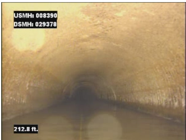
Photo: 008390_D_029378_SRV_212.jpg, VCR No.: 1 212FT, Surface Reinforcement Visible, from 08 to 04 o'clock, within 8 inches of joint: NO, Finish
