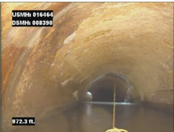
Photo: 016464_D_008390_IS_972.jpg, VCR No.: 1 972FT, Infiltration Stain, from 08 to 04 o'clock, within 8 inches of joint: YES
