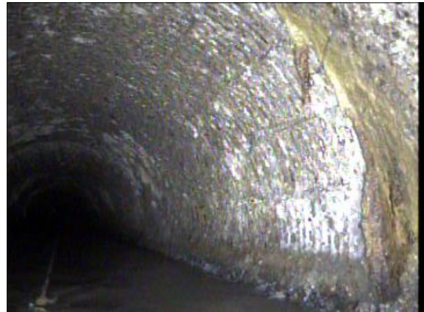
Photo: PWC-2103892-01-AMH '008396'-AMH '008397'-IS at 245.4 ft.JPG, 00:10:37 245.4FT, Infiltration Stain, from 02 to 04 o'clock, within 8 inches: NO
