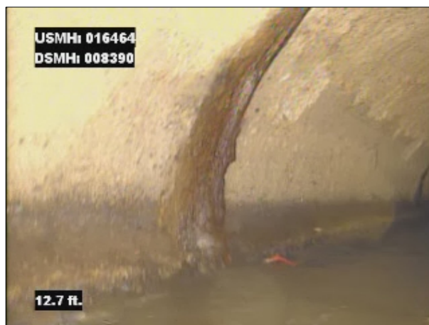
Photo: 016464_D_008390_DAE_13.jpg, VCR No.: 1 13FT, Deposits Attached Encrustation, 5 %of cross sectional area, from 07 to 05 o'clock, , within 8 inches of joint: YES
