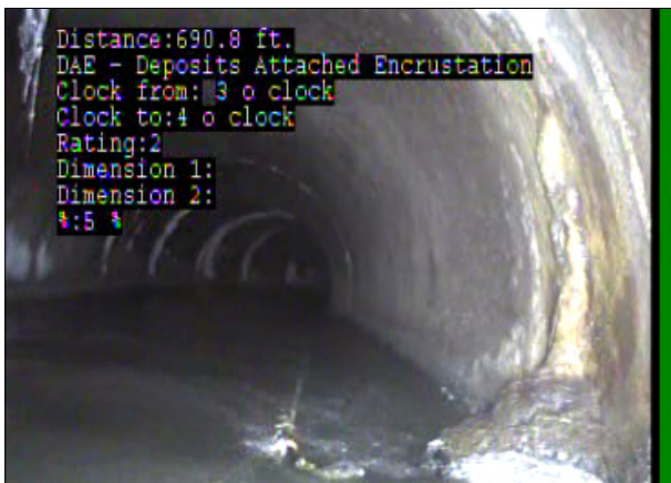
Photo: 016462_D_016461_DAE_690.8_46_A.jpg, 00:40:07 690.8FT, Deposits Attached Encrustation, 5% of cross sectional area, from 03 to 04 o'clock, within 8 inches: NO
