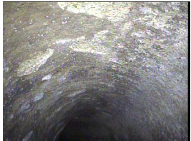
Photo: PWC-2103892-01-AMH '008397'-AMH '016462'-LL at 212.1 ft.JPG, 00:12:15 212.1FT, Alignment Left, 25°
