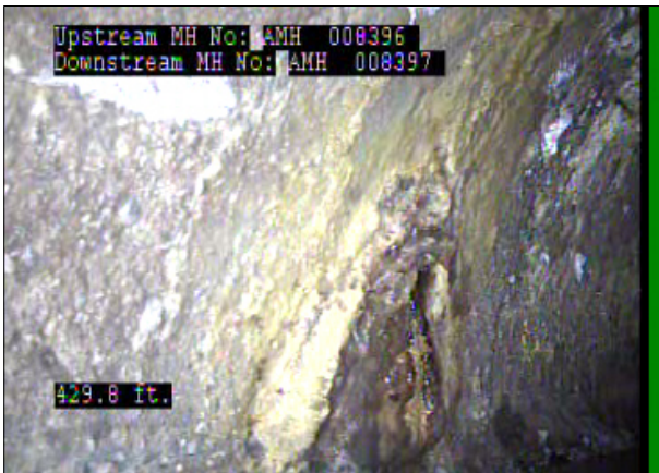
Photo: 008396_D_008397_IS_429.8_15_A.jpg, 00:22:25 429.8FT, Infiltration Stain, at 08 o'clock, within 8 inches: NO
