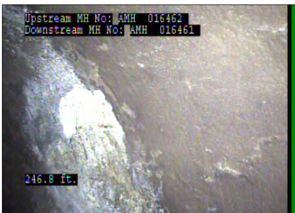
Photo: 016462_D_016461_SSS_246.8_35_A.jpg, 00:10:26 246.8FT, Surface Spalling, from 08 to 04 o'clock, within 8 inches: NO
