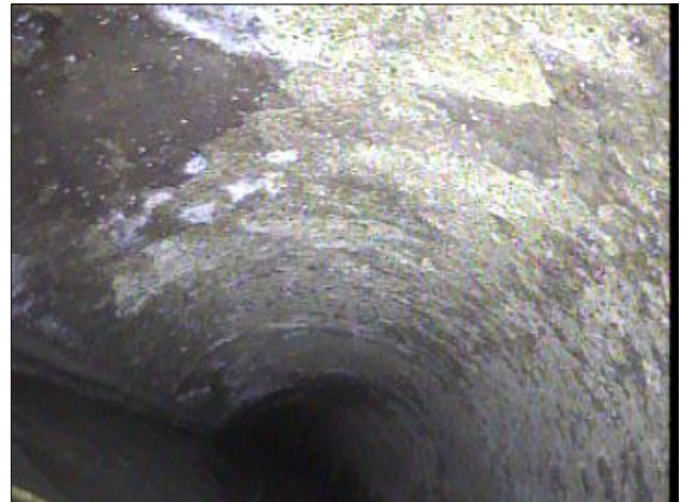
Photo: PWC-2103892-01-AMH '008397'-AMH '016462'-LL at 169.8 ft.JPG, 00:10:03 169.8FT, Alignment Left, 25°
