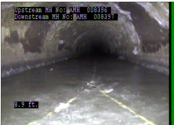
Photo: 008396_D_008397_SRC_8.9_8_A.jpg, 00:00:51 8.9FT, Surface Reinforcement Corroded, from 09 to 03 o'clock, within 8 inches: NO
