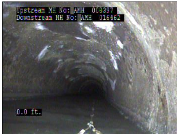
Photo: PWC-2103892-01-AMH '008397'-AMH '016462'-MWL at 0.0 ft.JPG OFT, Water Level, 50% of cross sectional area
