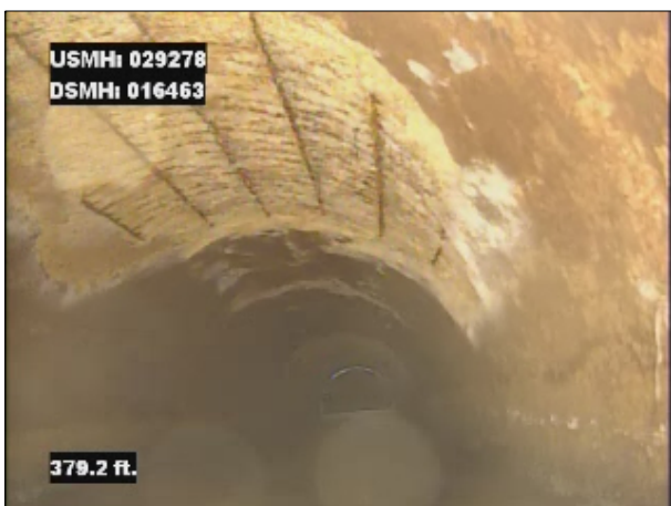
Photo: 029378_D_016463_SRV_379.jpg, VCR No.: 1 379FT, Surface Reinforcement Visible, from 10 to 02 o'clock, within 8 inches of joint: NO
