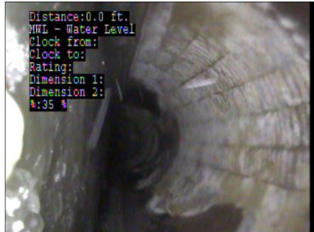
Photo: PWC-2103892-01-AMH '016461'-AMH '016460'-MWL at 0.0 ft.JPG OFT, Water Level, 35% of cross sectional area
