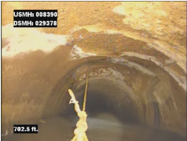
Photo: 008390_D_029378_SAV_702.5.jpg, VCR No.: 1 702.5FT, Surface Aggregate Visible, from 07 to 05 o'clock, within 8 inches of joint: YES, Finish
