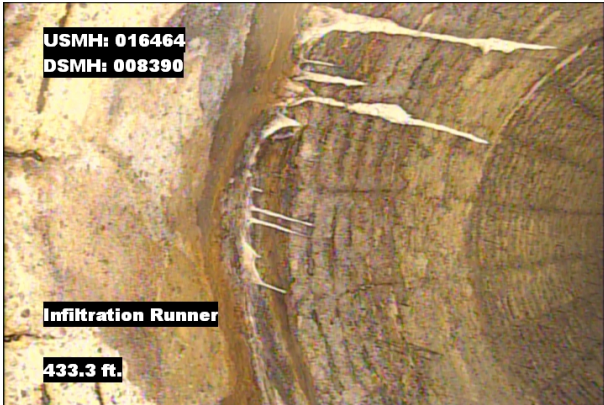
Photo: 016464_D_008390_IR_433.3.jpg, VCR No.: 1 433.3FT, Infiltration Runner, from 11 to 10 o'clock, within 8 inches: YES
