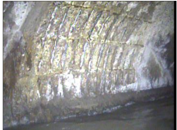
Photo: PWC-2103892-01-AMH '016462'-AMH '016461'-SRC at 508.4 ft.JPG, 00:26:52 508.4FT, Surface Reinforcement Corroded, from 09 to 11 o'clock, within 8 inches: NO
