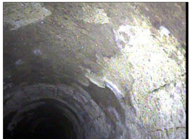
Photo: PWC-2103892-01-AMH '008397'-AMH '016462'-SRC at 93.5 ft.JPG, 00:05:10 93.5FT, Surface Reinforcement Corroded, from 08 to 04 o'clock, within 8 inches: NO
