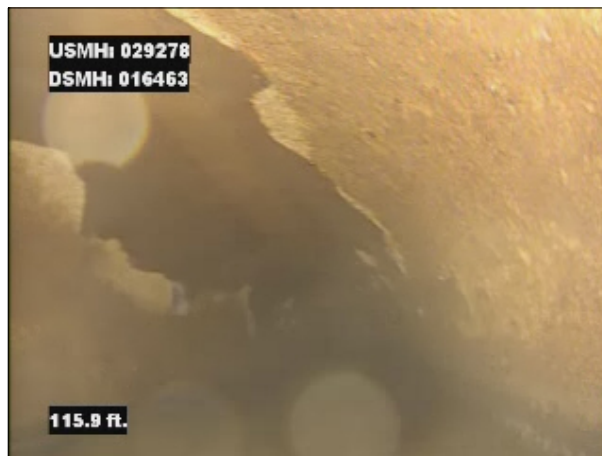
Photo: 029378_D_016463_SRV_115.jpg, VCR No.: 1 115FT, Surface Reinforcement Visible, from 08 to 04 o'clock, within 8 inches of joint: NO, Finish
