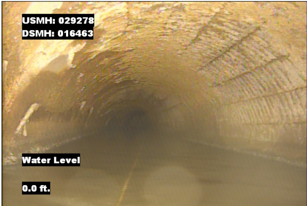
Photo: 029378_D_016463_MWL_0.jpg, VCR No.: 1 0FT, Water Level, 40% of cross sectional area
