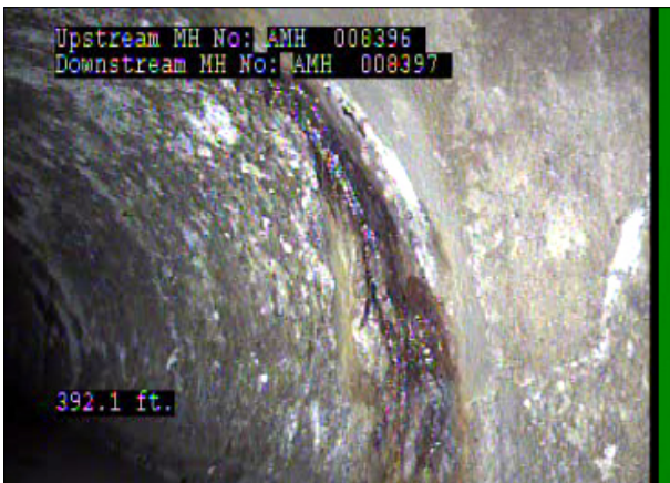
Photo: 008396_D_008397_IS_392_14_A.jpg, 00:20:09 392FT, Infiltration Stain, from 01 to 04 o'clock, within 8 inches: NO
