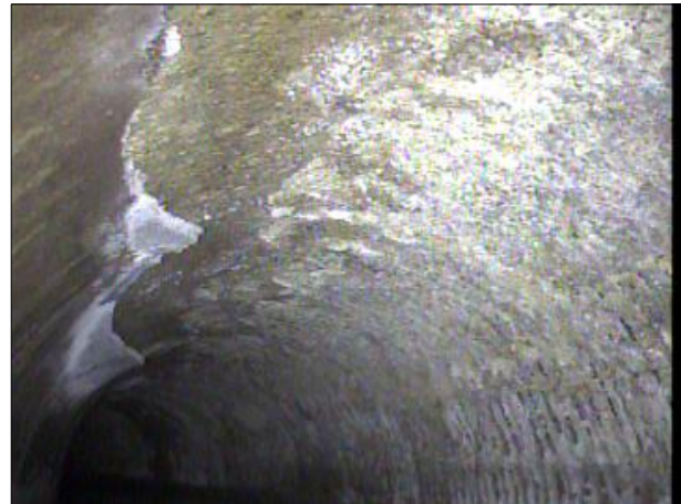
Photo: PWC-2103892-01-AMH '008397'-AMH '016462'-LL at 246.7 ft.JPG, 00:15:08 246.7FT, Alignment Left, 25°
