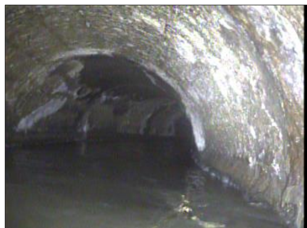
Photo: PWC-2103892-01-AMH '016462'-AMH '016461'-LR at 478.3 ft.JPG, 00:24:03 478.3FT, Alignment Right, 25°
