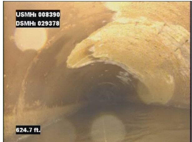
Photo: 008390_D_029378_SRV_624.jpg, VCR No.: 1 624FT, Surface Reinforcement Visible, from 01 to 04 o'clock, within 8 inches of joint: NO
