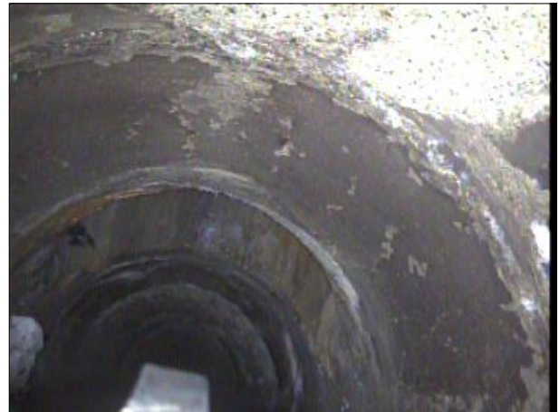
Photo: PWC-2103892-01-AMH '016463'-AMH '008396'-SRP at 840.0 ft.JPG, 03:06:49 840FT, Surface Reinforcement Projecting, from 09 to 03 o'clock, within 8 inches: NO
