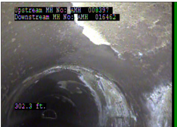
Photo: 008397_D_016462_SRC_302.1_29_A.jpg, 00:18:46 302.1FT, Surface Reinforcement Corroded, from 08 to 04 o'clock, within 8 inches: NO
