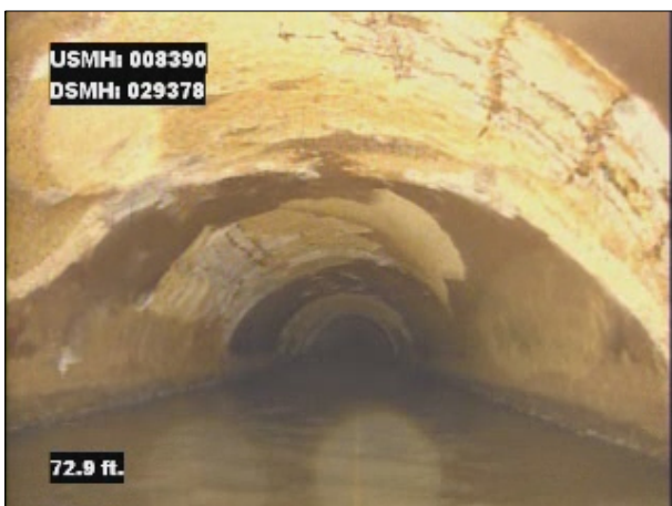
Photo: 008390_D_029378_SRV_72.9.jpg, VCR No.: 1 72.9FT, Surface Reinforcement Visible, from 08 to 04 o'clock, within 8 inches of joint: NO, Start
