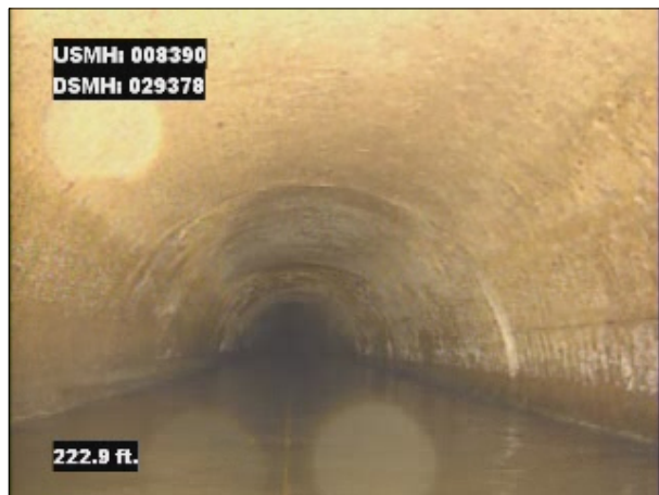
Photo: 008390_D_029378_SAV_222.jpg, VCR No.: 1 222FT, Surface Aggregate Visible, from 07 to 05 o'clock, within 8 inches of joint: YES, Start
