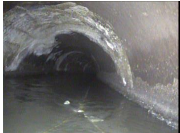
Photo: PWC-2103892-01-AMH '016462'-AMH '016461'-LR at 591.8 ft.JPG, 00:33:50 591.8FT, Alignment Right, 20°
