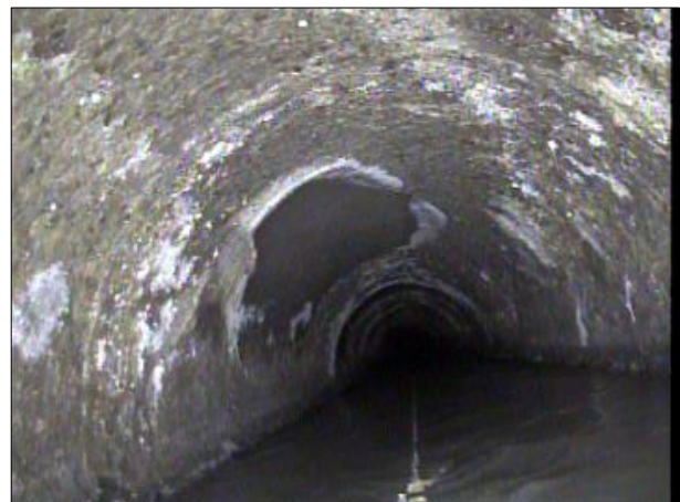
Photo: PWC-2103892-01-AMH '008396'-AMH '008397'-SRC at 364.5 ft.JPG, 00:17:29 364.5FT, Surface Reinforcement Corroded, from 09 to 03 o'clock, within 8 inches: NO
