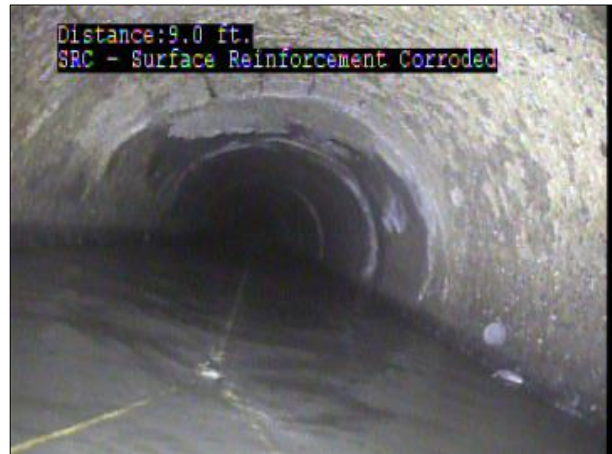
Photo: PWC-2103892-01-AMH '016462'-AMH '016461'-SRC at 9.0 ft.JPG, 00:00:31 9FT, Surface Reinforcement Corroded, at 12 o'clock, within 8 inches: NO
