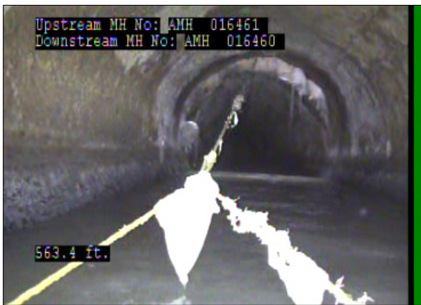
Photo: 016461_D_016460_SRC_563.4_56_A.jpg, 00:27:26 563.4FT, Surface Reinforcement Corroded, from 09 to 03 o'clock, within 8 inches: NO
