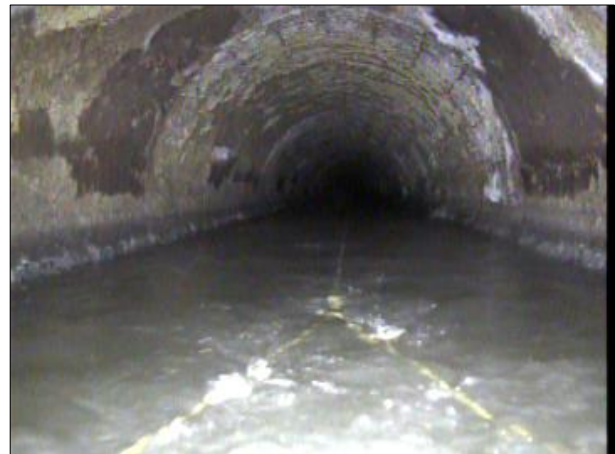
Photo: PWC-2103892-01-AMH '008396'-AMH '008397'-SRC at 8.9 ft.JPG, 00:00:51 8.9FT, Surface Reinforcement Corroded, from 09 to 03 o'clock, within 8 inches: NO
