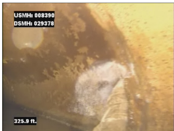
Photo: 008390_D_029378_DAR_325.jpg, VCR No.: 1 325FT, Deposits Attached Ragging, 5 %of cross sectional area, from 03 to 04 o'clock, , within 8 inches of joint: YES
