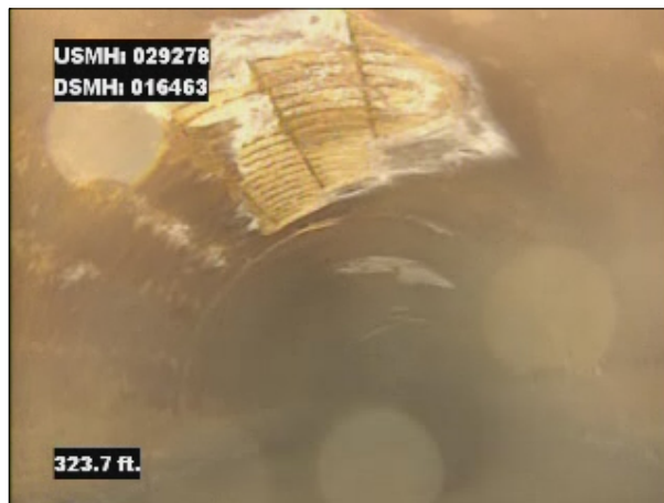
Photo: 029378_D_016463_SRV_323.jpg, VCR No.: 1 323FT, Surface Reinforcement Visible, from 10 to 01 o'clock, within 8 inches of joint: NO
