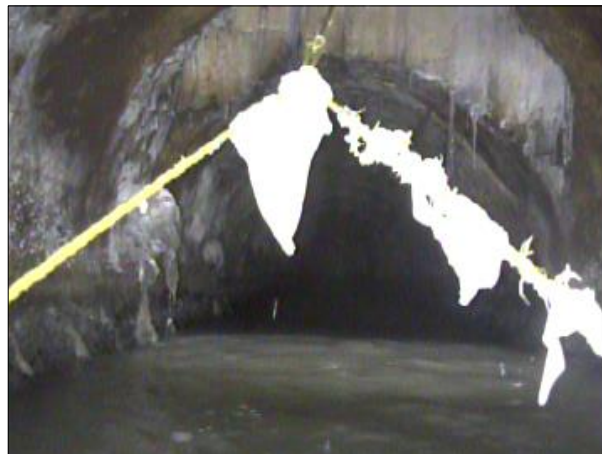
Photo: PWC-2103892-01-AMH '016461'-AMH '016460'-SRC at 563.4 ft.JPG, 00:27:26 563.4FT, Surface Reinforcement Corroded, from 09 to 03 o'clock, within 8 inches: NO
