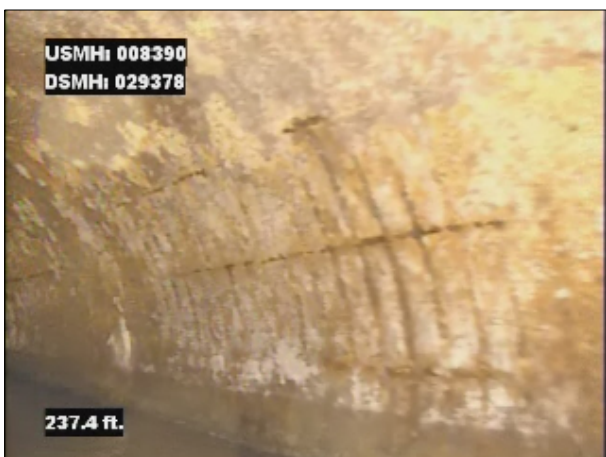
Photo: 008390_D_029378_SRV_237.jpg, VCR No.: 1 237FT, Surface Reinforcement Visible, from 08 to 04 o'clock, within 8 inches of joint: NO, Start
