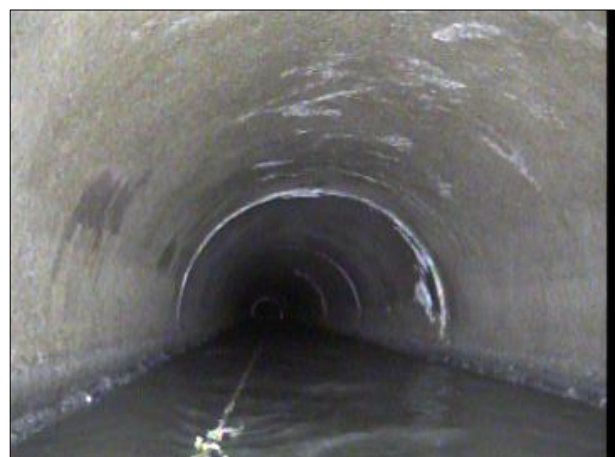
Photo: PWC-2103892-01-AMH '008396'-AMH '008397'-SAP at 511.4 ft.JPG, 00:27:08 511.4FT, Surface Aggregate Projecting, from 09 to 03 o'clock, within 8 inches of joint: NO, Finish
