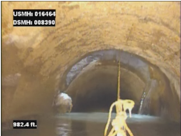
Photo: 016464_D_008390_SRV_982.jpg, VCR No.: 1 982FT, Surface Reinforcement Visible, from 08 to 04 o'clock, within 8 inches of joint: YES, Finish
