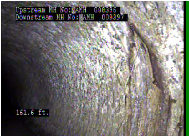
Photo: 008396_D_008397_IR_161.5_9_A.jpg, 00:06:41 161.5FT, Infiltration Runner, from 02 to 03 o'clock, within 8 inches: NO
