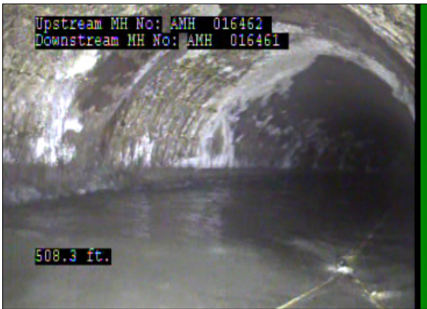
Photo: 016462_D_016461_SRC_508.4_40_A.jpg, 00:26:52 508.4FT, Surface Reinforcement Corroded, from 09 to 11 o'clock, within 8 inches: NO
