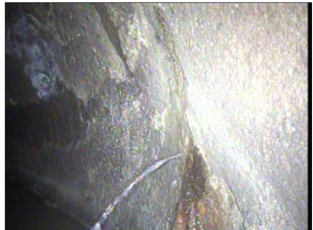
Photo: PWC-2103892-01-AMH '016462'-AMH '016461'-IR at 557.5 ft.JPG, 00:31:52 557.5FT, Infiltration Runner, at 03 o'clock, within 8 inches: NO
