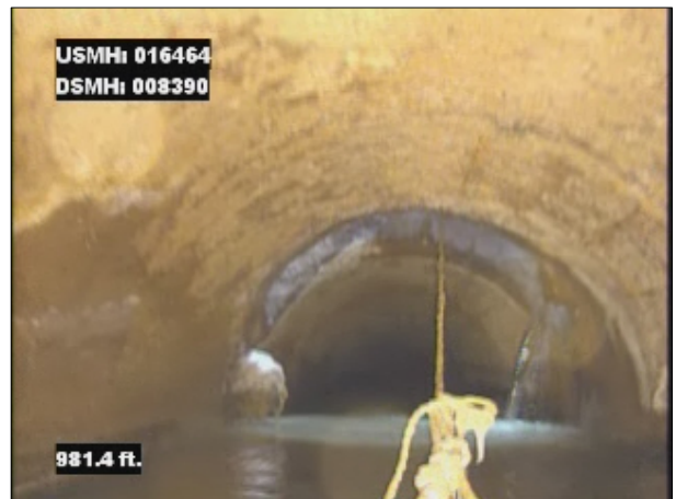
Photo: 016464_D_008390_SAV_981.jpg, VCR No.: 1 981FT, Surface Aggregate Visible, from 07 to 05 o'clock, within 8 inches of joint: YES, Finish
