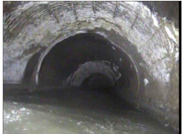
Photo: PWC-2103892-01-AMH '016462'-AMH '016461'-SSS at 789.7 ft.JPG, 00:45:32 789.7FT, Surface Spalling, from 08 to 04 o'clock, within 8 inches: NO
