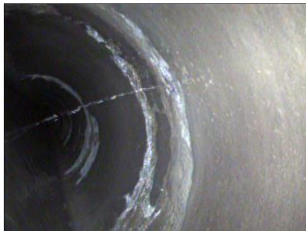
Photo: PWC-2103892-01-AMH '016462'-AMH '016461'-IR at 365.7 ft.JPG, 00:18:26 365.7FT, Infiltration Runner, at 12 o'clock, within 8 inches: NO
