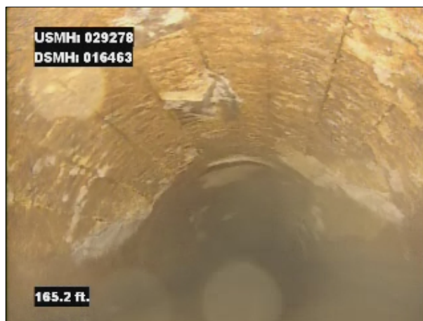
Photo: 029378_D_016463_SRV_165.jpg, VCR No.: 1 165FT, Surface Reinforcement Visible, from 08 to 04 o'clock, within 8 inches of joint: NO
