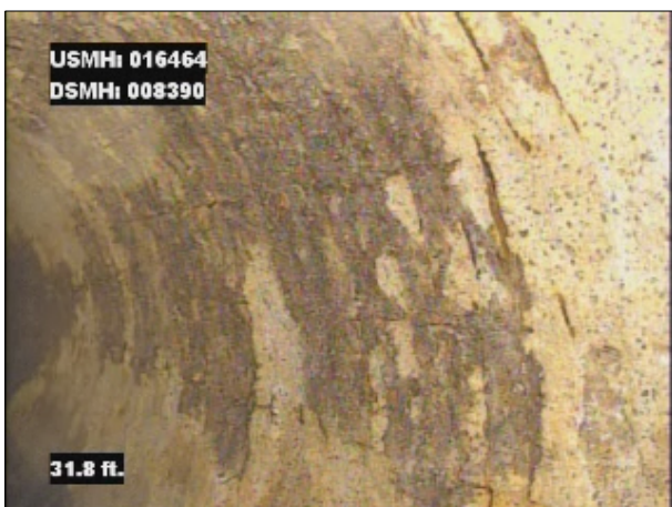
Photo: 016464_D_008390_SRV_31.jpg, VCR No.: 1 31FT, Surface Reinforcement Visible, from 08 to 04 o'clock, within 8 inches of joint: NO, Start
