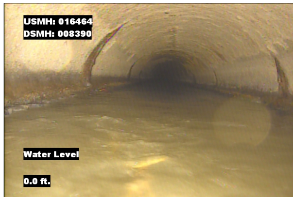
Photo: 016464_D_008390_MWL_0.jpg, VCR No.: 1 0FT, Water Level, 45% of cross sectional area
