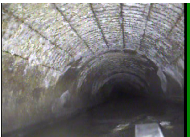
Photo: 016463_D_008396_SRP_0_3_A.jpg, 00:00:22 OFT, Surface Reinforcement Projecting, from 09 to 03 o'clock, within 8 inches: NO
