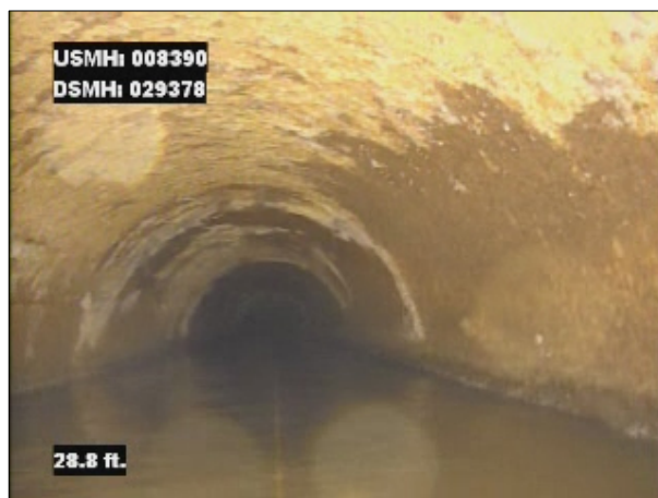
Photo: 008390_D_029378_SRV_28.7.jpg, VCR No.: 1 28.7FT, Surface Reinforcement Visible, from 08 to 04 o'clock, within 8 inches of joint: NO, Finish
