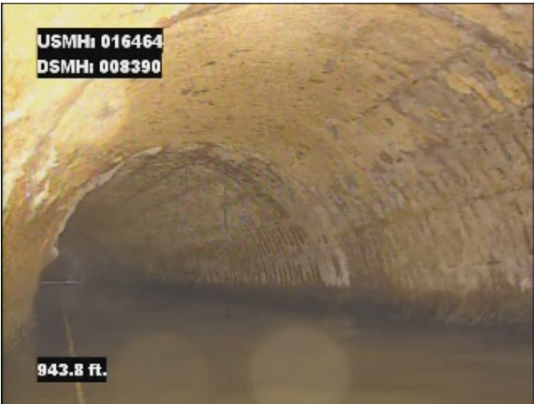
Photo: 016464_D_008390_SRV_943.jpg, VCR No.: 1 943FT, Surface Reinforcement Visible, from 08 to 04 o'clock, within 8 inches of joint: YES, Start
