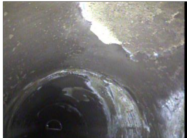
Photo: PWC-2103892-01-AMH '008397'-AMH '016462'-SRC at 302.1 ft.JPG, 00:18:46 302.1FT, Surface Reinforcement Corroded, from 08 to 04 o'clock, within 8 inches: NO
