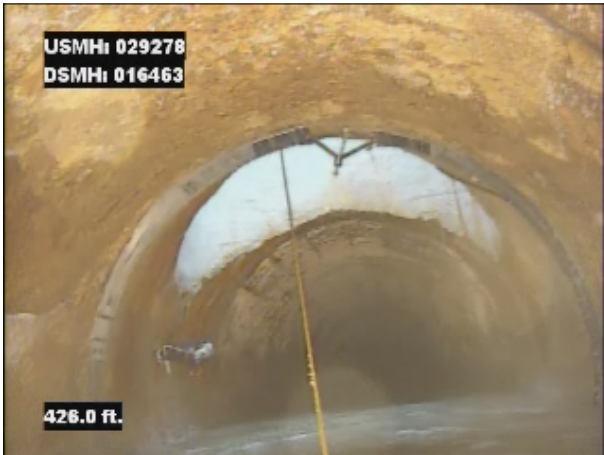
Photo: 029378_D_016463_SAV_426.jpg, VCR No.: 1 426FT, Surface Aggregate Visible, from 08 to 04 o'clock, within 8 inches of joint: NO, Finish
