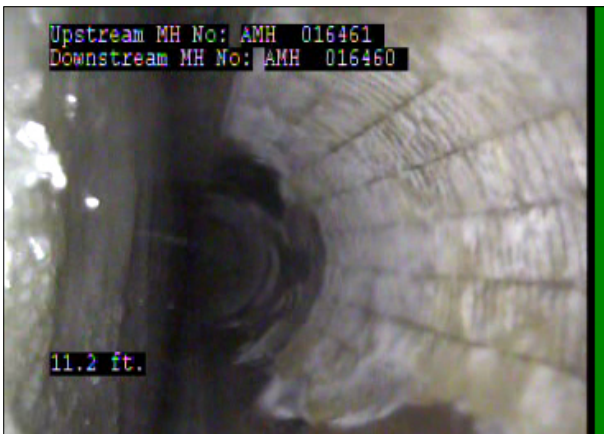
Photo: 016461_D_016460_SRC_11.2_53_A.jpg, 00:00:45 11.2FT, Surface Reinforcement Corroded, from 09 to 03 o'clock, within 8 inches: NO
