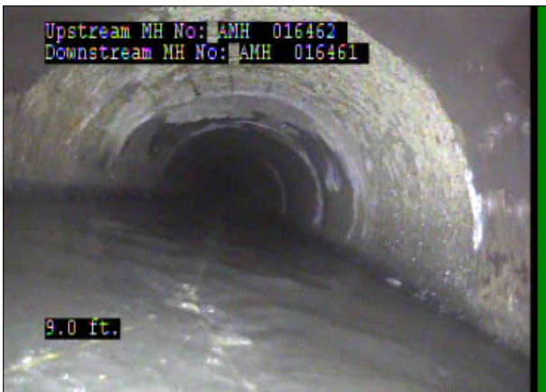
Photo: 016462_D_016461_SRC_9_33_A.jpg, 00:00:31 9FT, Surface Reinforcement Corroded, at 12 o'clock, within 8 inches: NO
