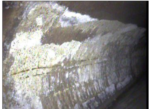
Photo: PWC-2103892-01-AMH '016462'-AMH '016461'-SRC at 544.8 ft.JPG, 00:30:28 544.8FT, Surface Reinforcement Corroded, from 08 to 11 o'clock, within 8 inches: NO
