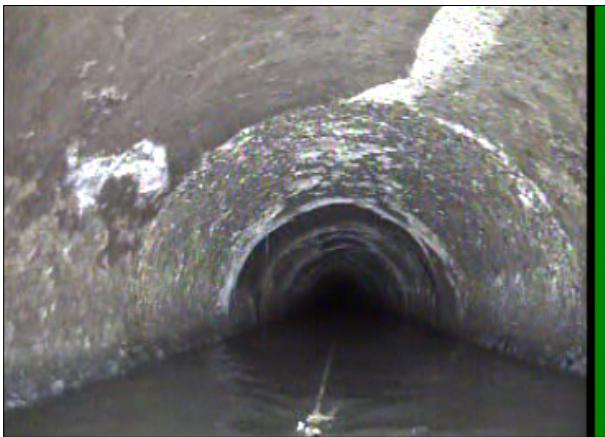
Photo: 008396_D_008397_SAP_367.1_13_A.jpg, 00:18:42 367.1FT, Surface Aggregate Projecting, from 09 to 03 o'clock, within 8 inches: NO
