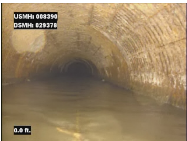
Photo: 008390_D_029378_SRV_0.1.jpg, VCR No.: 1 0.1FT, Surface Reinforcement Visible, from 08 to 04 o'clock, within 8 inches of joint: NO, Start
