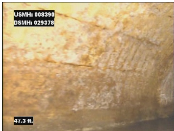
Photo: 008390_D_029378_SRV_47.3.jpg, VCR No.: 1 47.3FT, Surface Reinforcement Visible, from 08 to 12 o'clock, within 8 inches of joint: YES
