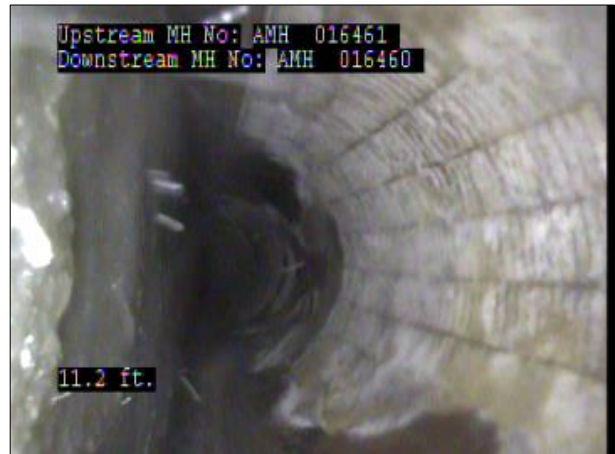
Photo: PWC-2103892-01-AMH '016461'-AMH '016460'-SRC at 11.2 ft.JPG, 00:00:45 11.2FT, Surface Reinforcement Corroded, from 09 to 03 o'clock, within 8 inches: NO
