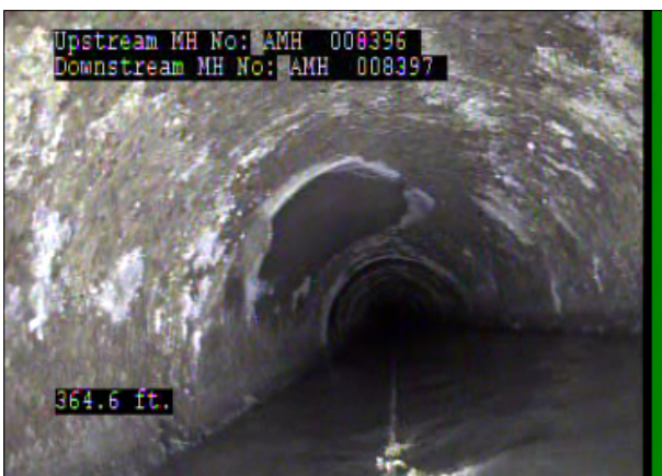
Photo: 008396_D_008397_SRC_364.5_12_A.jpg, 00:17:29 364.5FT, Surface Reinforcement Corroded, from 09 to 03 o'clock, within 8 inches: NO
