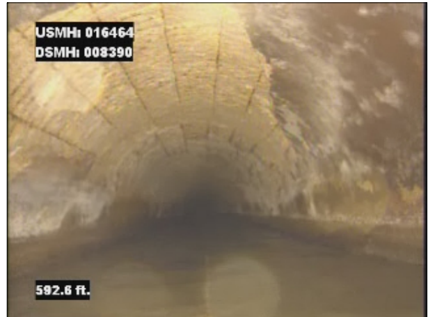
Photo: 016464_D_008390_SRV_592.jpg, VCR No.: 1 592FT, Surface Reinforcement Visible, from 08 to 04 o'clock, within 8 inches of joint: NO, Start
