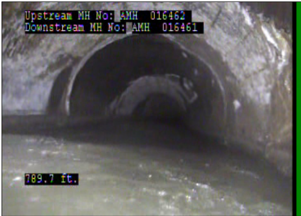
Photo: 016462_D_016461_SSS_789.7_48_A.jpg, 00:45:32 789.7FT, Surface Spalling, from 08 to 04 o'clock, within 8 inches: NO
