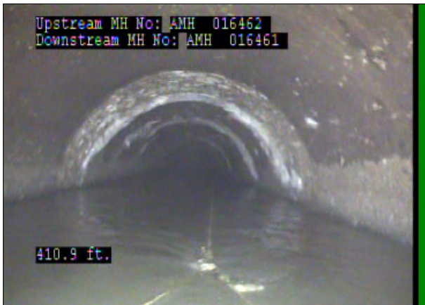
Photo: 016462_D_016461_SRI_410.2_38_A.jpg, 00:20:37 410.2FT, Surface Roughness Increased, from 08 to 04 o'clock, within 8 inches: NO
