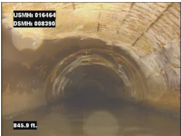
Photo: 016464_D_008390_SRV_845.jpg, VCR No.: 1 845FT, Surface Reinforcement Visible, from 11 to 04 o'clock, within 8 inches of joint: YES
