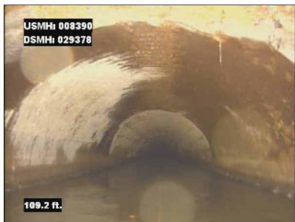
Photo: 008390_D_029378_SAV_109.2.jpg, VCR No.: 1 109.2FT, Surface Aggregate Visible, from 08 to 04 o'clock, within 8 inches of joint: NO, Finish
