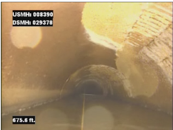
Photo: 008390_D_029378_SRV_675.jpg, VCR No.: 1 675FT, Surface Reinforcement Visible, from 08 to 04 o'clock, within 8 inches of joint: NO, Start
