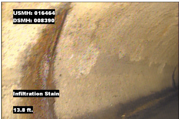
Photo: 016464_D_008390_IS_13.8.jpg, VCR No.: 1 13.8FT, Infiltration Stain, from 08 to 10 o'clock, within 8 inches: YES
