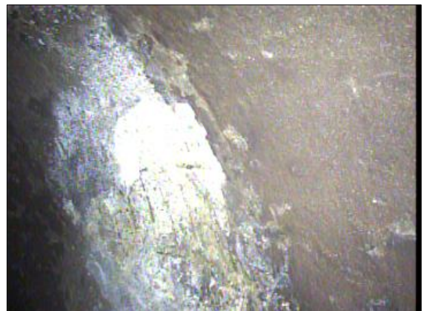
Photo: PWC-2103892-01-AMH '016462'-AMH '016461'-SSS at 246.8 ft.JPG, 00:10:26 246.8FT, Surface Spalling, from 08 to 04 o'clock, within 8 inches: NO
