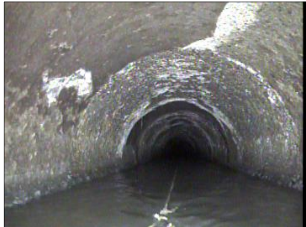
Photo: PWC-2103892-01-AMH '008396'-AMH '008397'-SAP at 367.1 ft.JPG, 00:18:42 367.1FT, Surface Aggregate Projecting, from 09 to 03 o'clock, within 8 inches: NO
