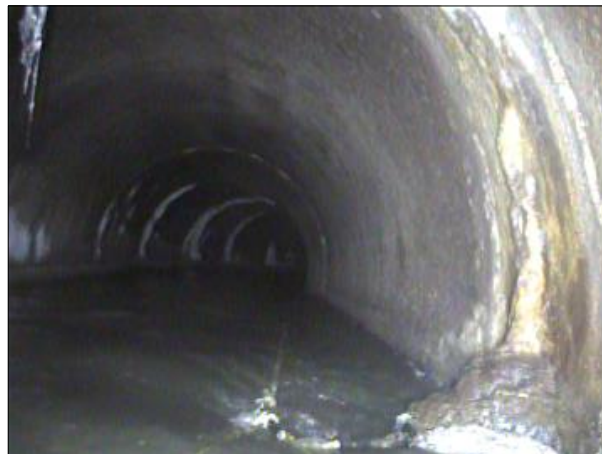
Photo: PWC-2103892-01-AMH '016462'-AMH '016461'-DAE at 690.8 ft.JPG, 00:40:07 690.8FT, Deposits Attached Encrustation, 5% of cross sectional area, from 03 to 04 o'clock, within 8 inches: NO
