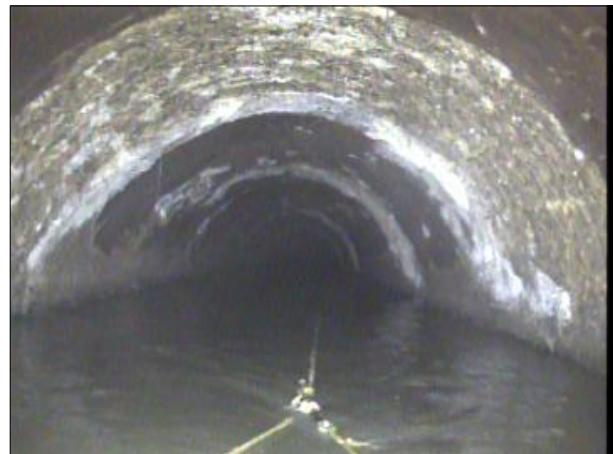
Photo: PWC-2103892-01-AMH '016462'-AMH '016461'-SRI at 410.2 ft.JPG, 00:20:37 410.2FT, Surface Roughness Increased, from 08 to 04 o'clock, within 8 inches: NO
