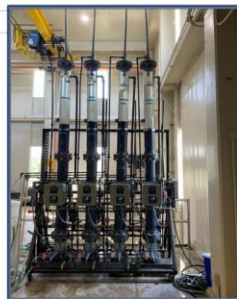
P.O Hoffer Pilot Test Columns
