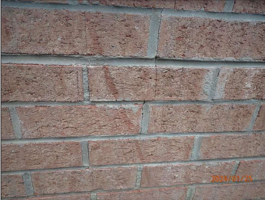
Photo 7 Step and vertical crack
