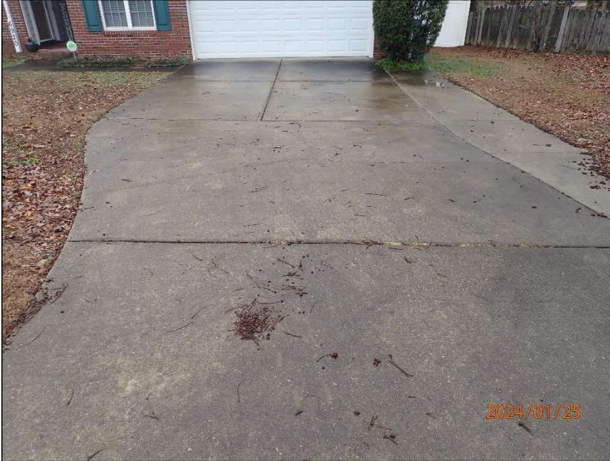
Photo 7 Cracks in concrete driveway
