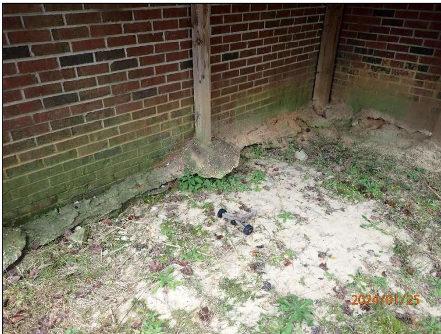
Photo 12 Potentially undermined foundation
