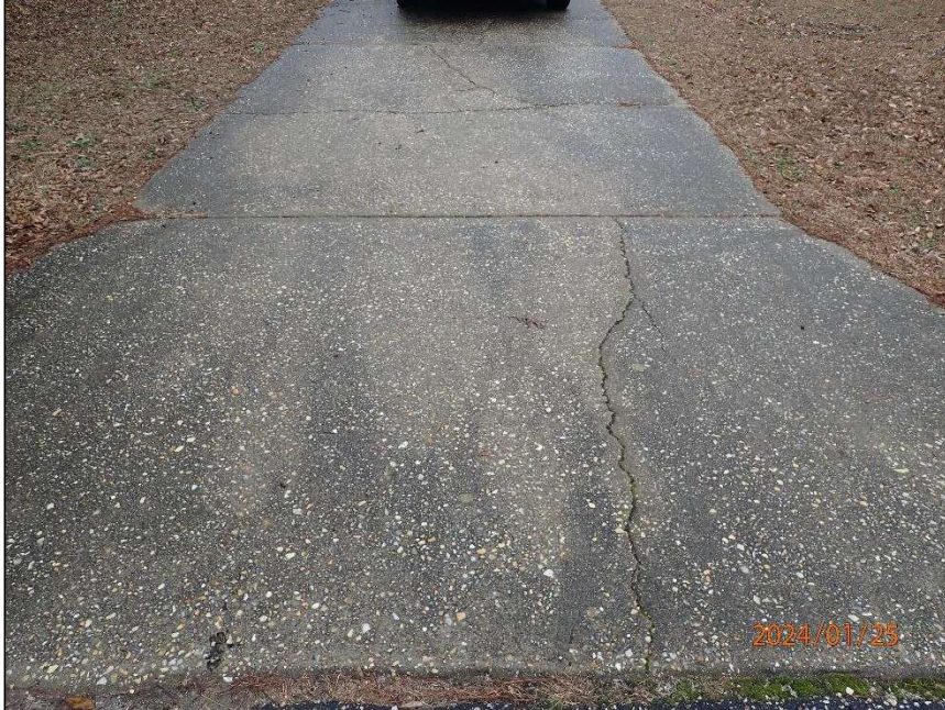
Photo 5 Cracks in concrete driveway
