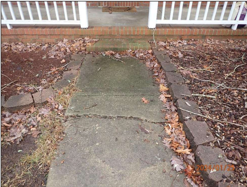
Photo 6 Cracks in concrete sidewalk
