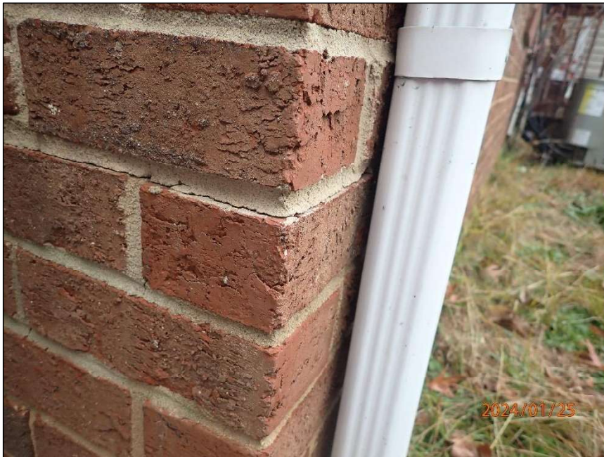
Photo 6 Step and horizontal crack
