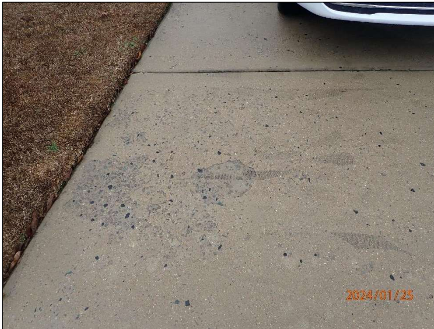
Photo 6 Cracks in concrete driveway and spalling
