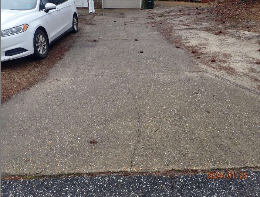
Photo 5 Cracks in concrete driveway
