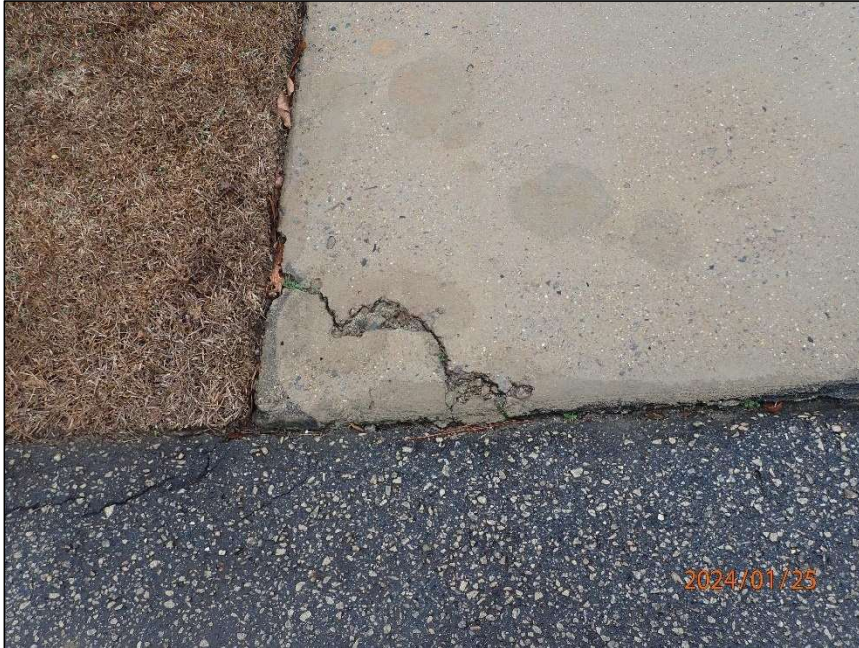
Photo 5 Cracks in concrete driveway - at corner
