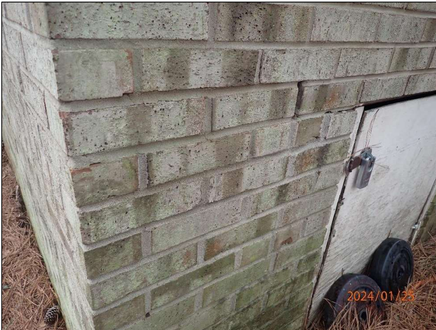
Photo 14 Horizontal and step crack
