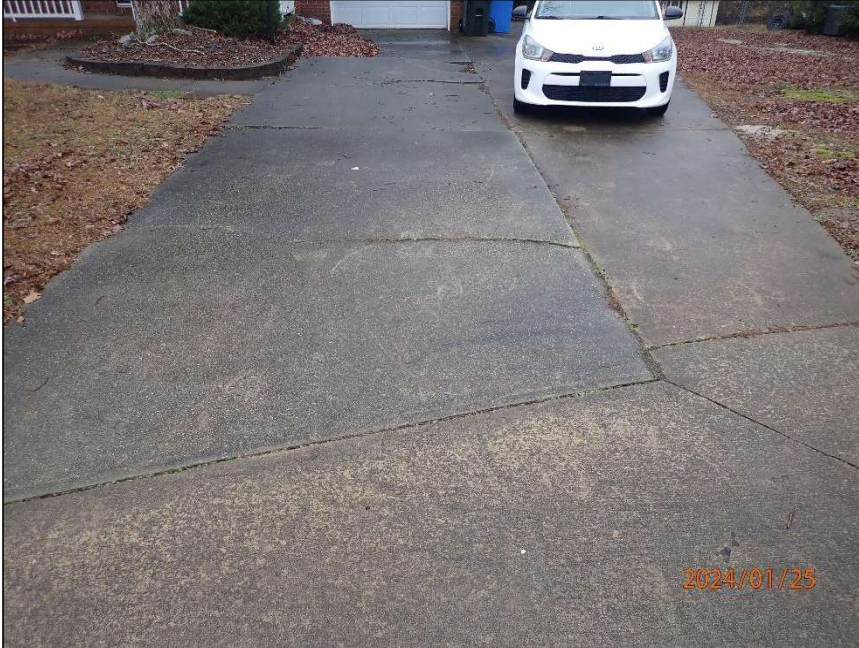
Photo 5 Cracks in concrete driveway
