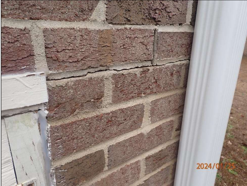
Photo 9 Step and Horizontal crack
