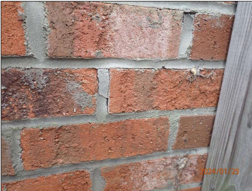
Photo 10 Horizontal and step crack
