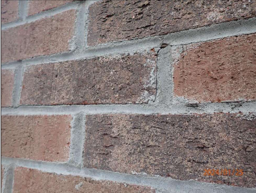
Photo 5 Horizontal and step crack
