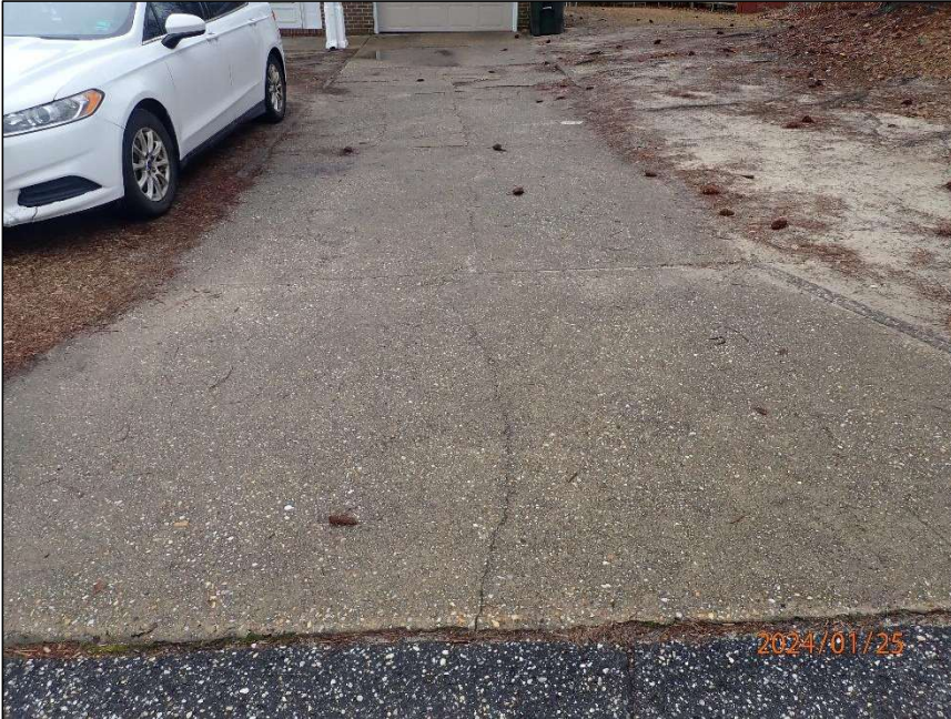
Photo 5 Cracks in concrete driveway
