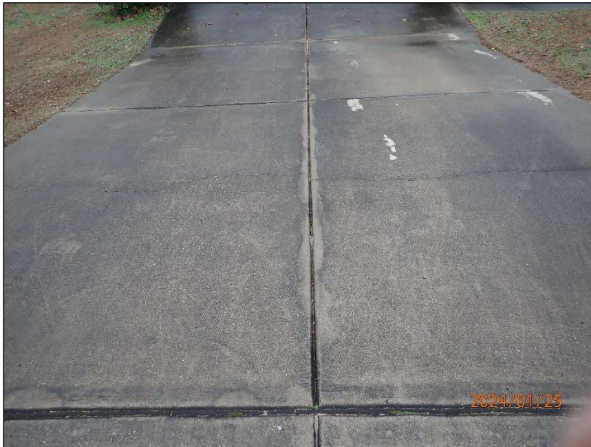
Photo 4 Cracks in concrete driveway
