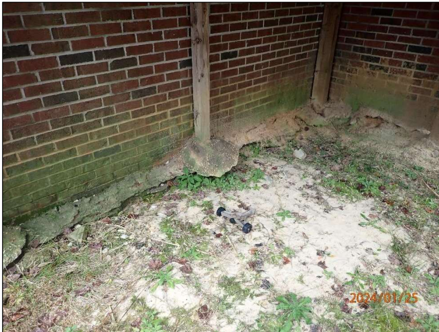
Photo 12 Potentially undermined foundation
