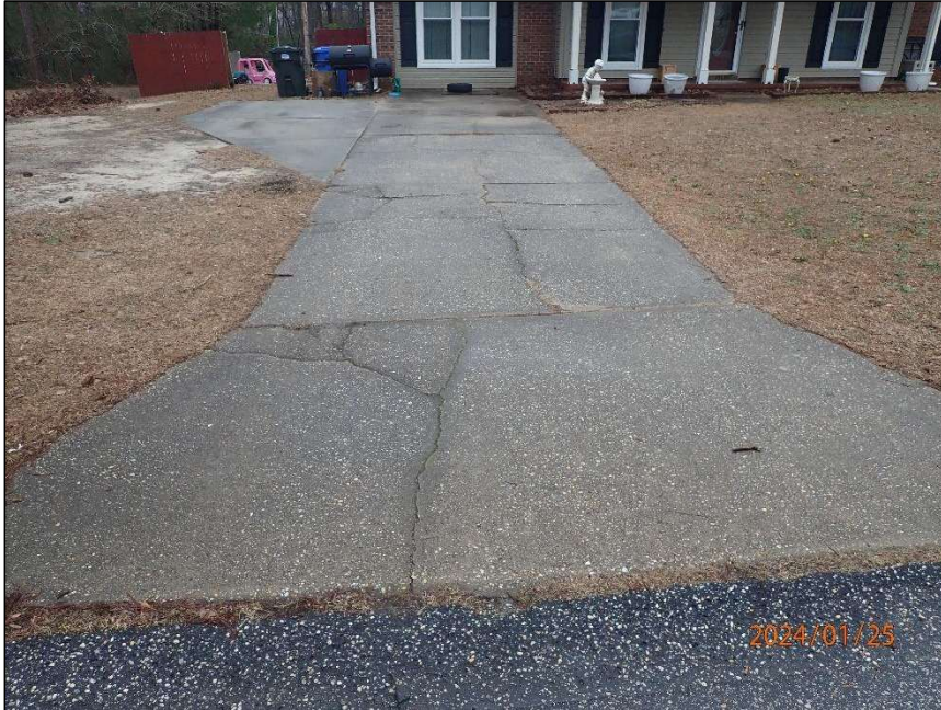
Photo 5 Cracks in concrete driveway
