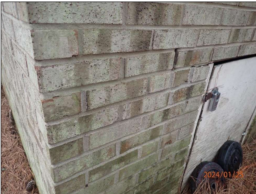
Photo 14 Horizontal and step crack
