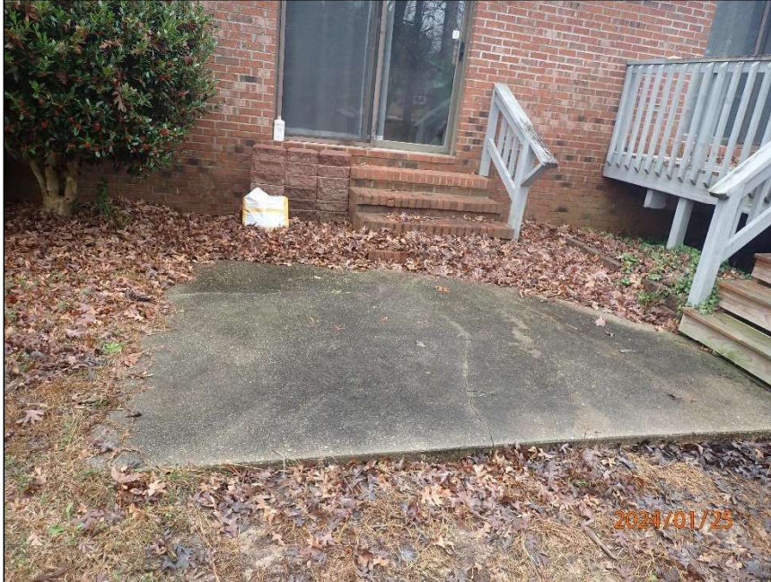
Photo 11 Cracks in concrete slab
