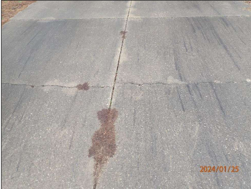
Photo 7 Cracks in concrete driveway
