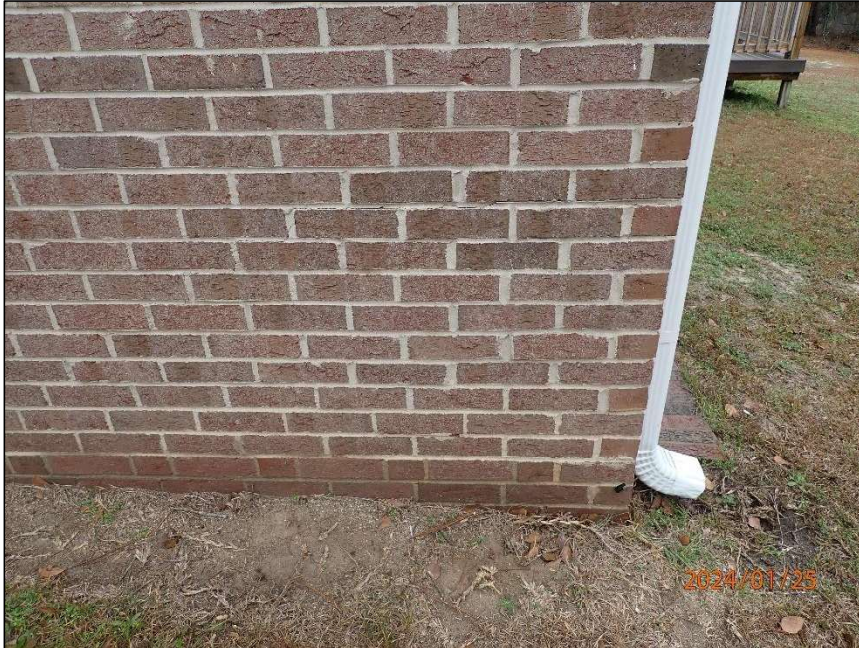
Photo 7 Step and Horizontal crack
