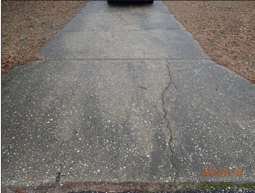
Photo 5 Cracks in concrete driveway
