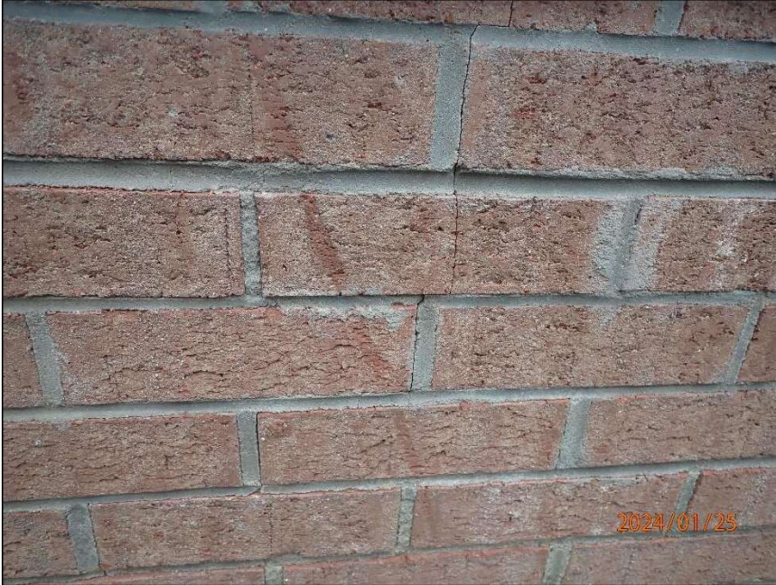
Photo 7 Step and vertical crack
