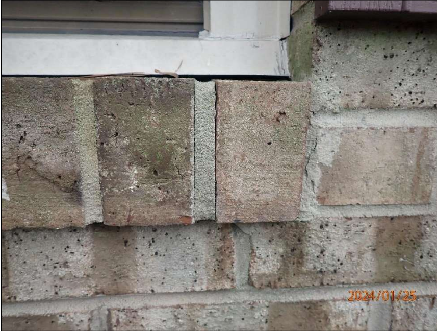
Photo 5 Displaced brick at window sill
