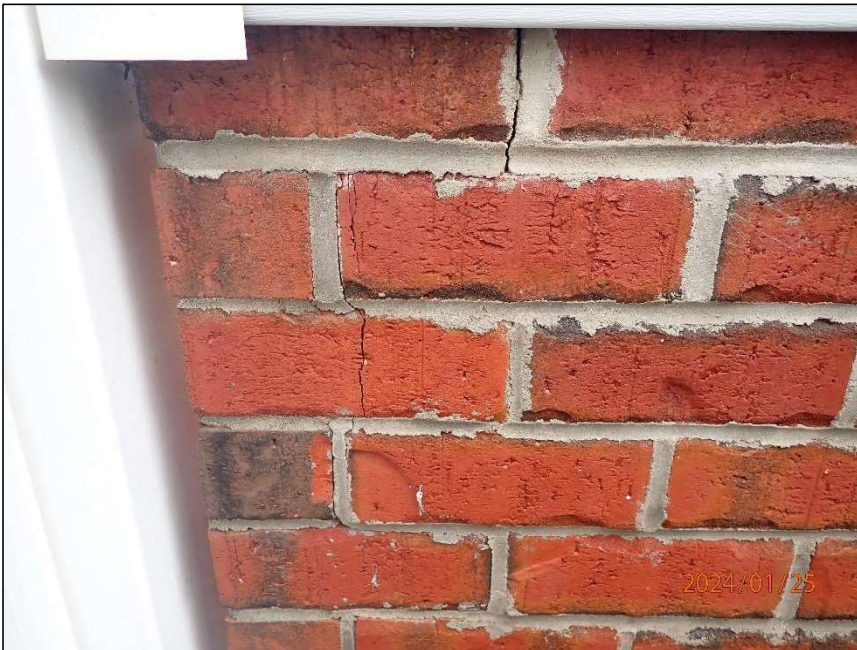
Photo 10 Step and vertical crack
